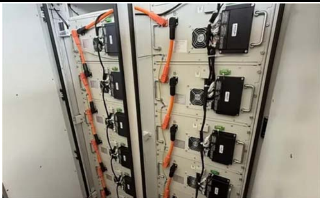
Figure 3: Amcharge Malaysia – BESS
